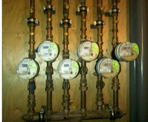
Manifold and Meters
